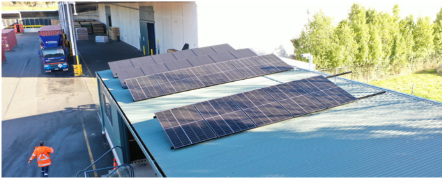
Solar panels recently installed at Port Otago's Sawyers Bay site as part of a solar power trial.
